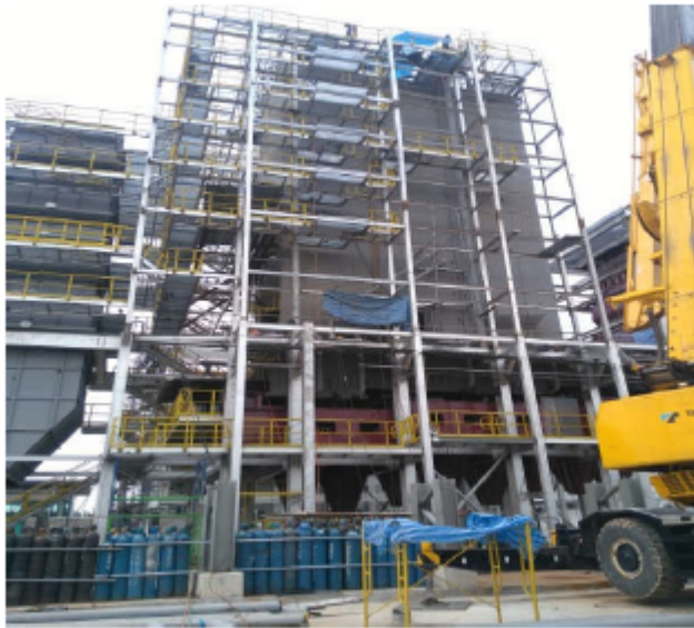
BIB for APCON / Thai - 2016 Bangkok Industrial Boiler 45 MWth, (42 bar, 420°C) grate combustion-system for RDF, Municipal + Industrial Waste
